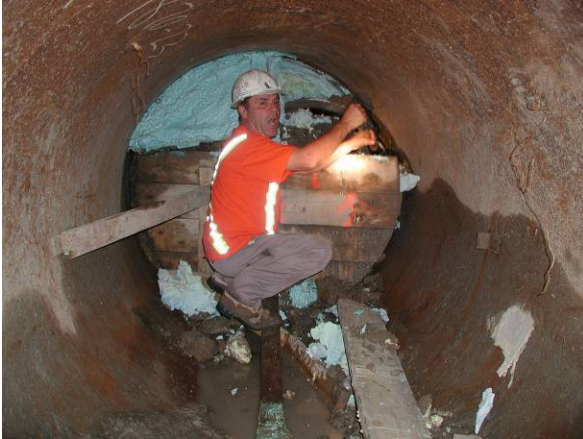
Figure 8 – Mine Bulkhead and Treating
